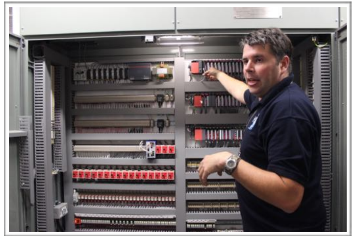
The new Nitrogen processing plant is fully automated and monitored via computer.
